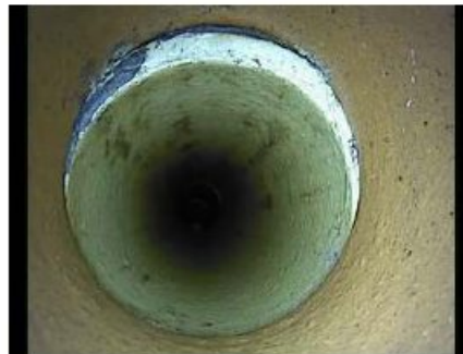
2) Medium Displaced Joint (from 12 o'clock to 4 o'clock)
