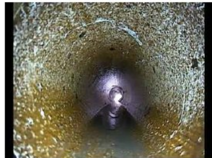
6) Crack (from 12 o'clock to 4 o'clock)
