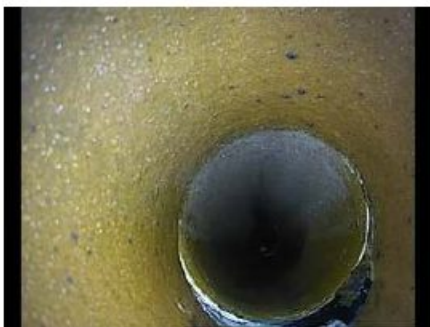
3) Crack at joint (from 12 o'clock to 4 o'clock)
