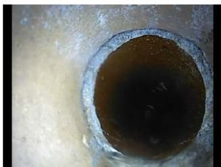
3) Medium Displaced Joint (from 12 o'clock to 4 o'clock)
