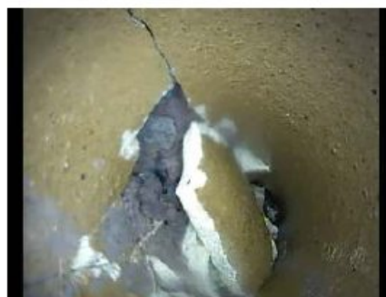
4) Hole in Pipework (from 12 o'clock to 4 o'clock)
