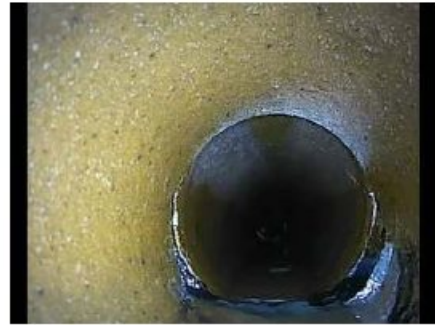
2) Crack at joint (from 12 o'clock to 4 o'clock)
