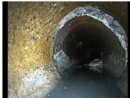
2) Medium Displaced Joint (from 12 o'clock to 4 o'clock)
