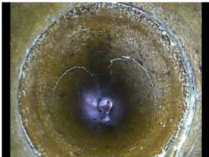
5) Crack (from 12 o'clock to 4 o'clock)
